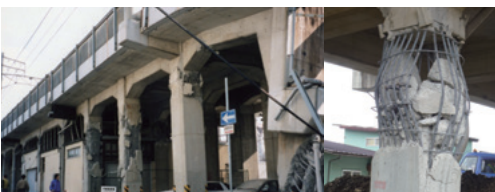
Field surveys on lifeline damages
