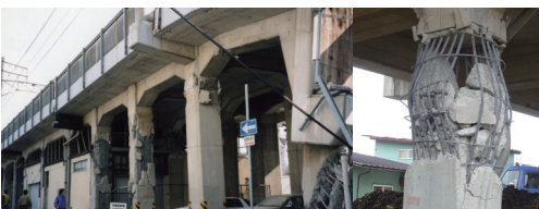
Field surveys on lifeline damages
