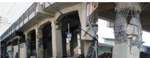
Field surveys on lifeline damages
